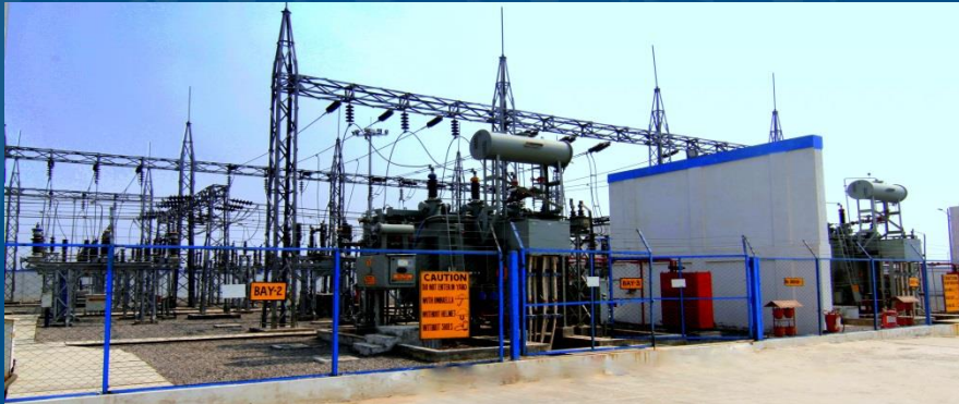
Tata Power - HT Substation
