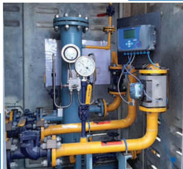
Replaced LPG with PNG for fuel efficiency at the Dadra Plant
