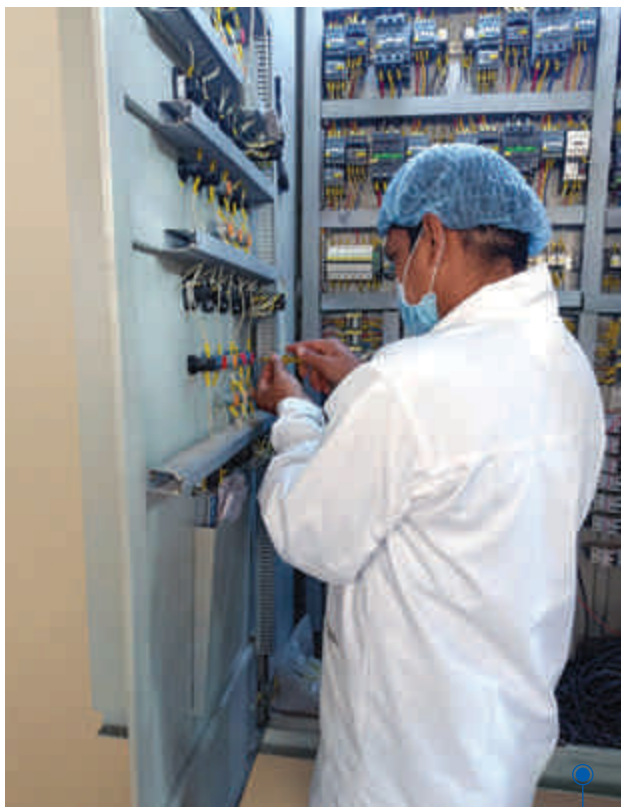
Blue Star's engineer resolving an electrical problem in the Cold Room control panel at Jubilant Commissory, Mumbai
