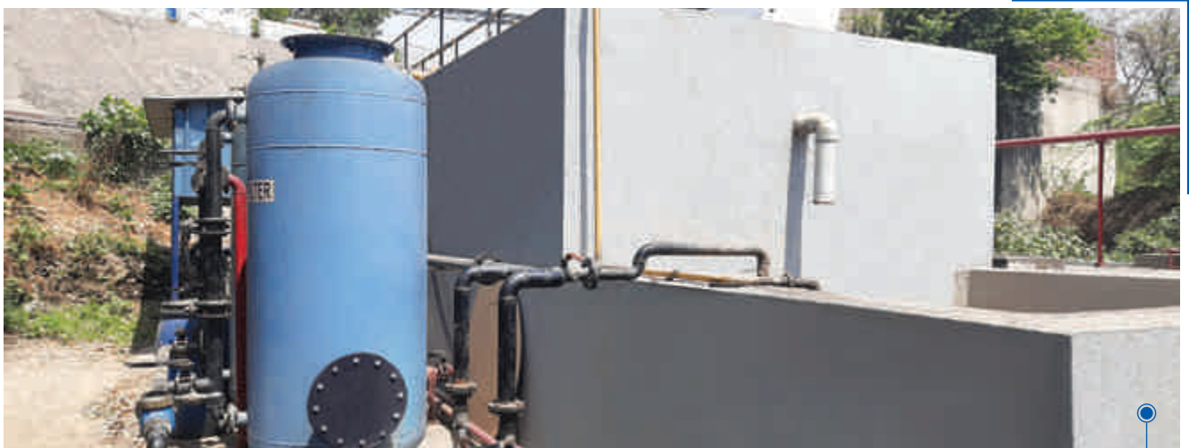
Water filtration plant at Blue Star's Himachal Pradesh manufacturing facility
