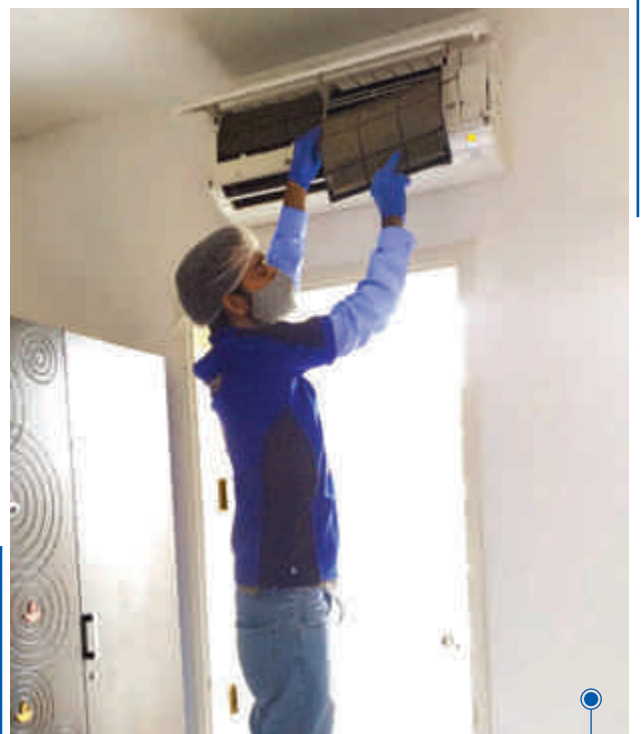
Blue Star's service technician servicing an air conditioner at a customer's residence
