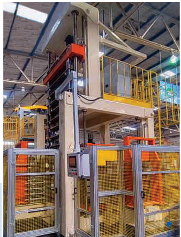
Vertical Expander installed at Blue Star's Himachal Pradesh Plant
