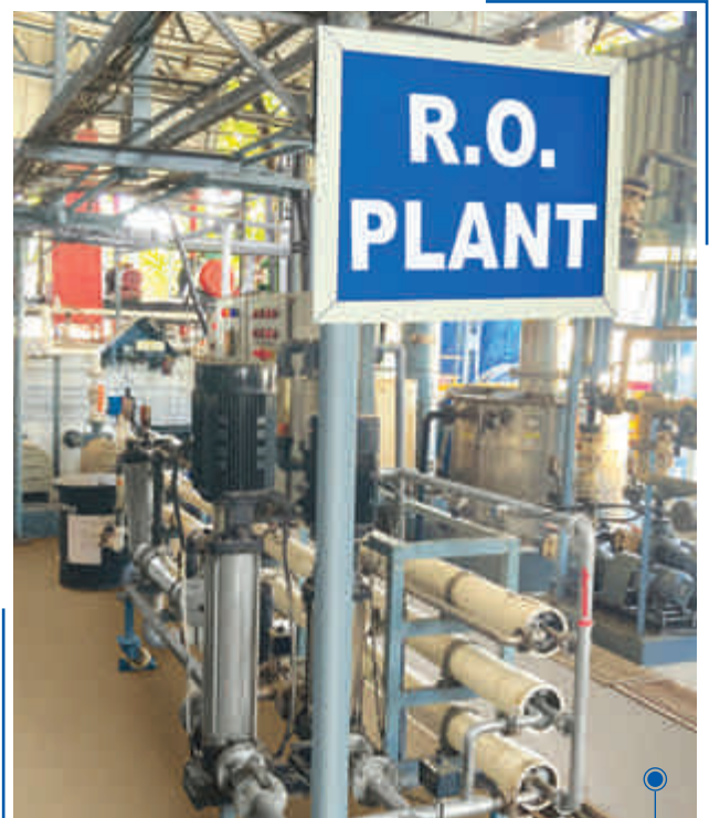
Reverse Osmosis (RO) Water Treatment Plant at Blue Star's Dadra manufacturing facility
