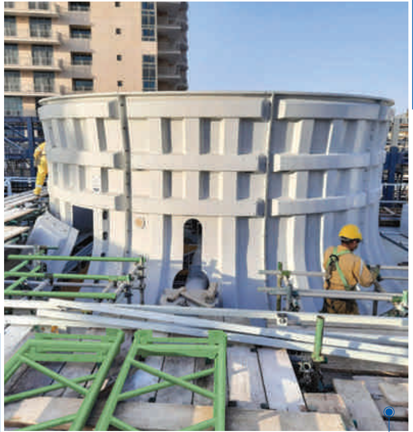
Cooling towers being installed by Blue Star at 'Gewan District Cooling Plant Project,' the Pearl-Doha, Qatar
