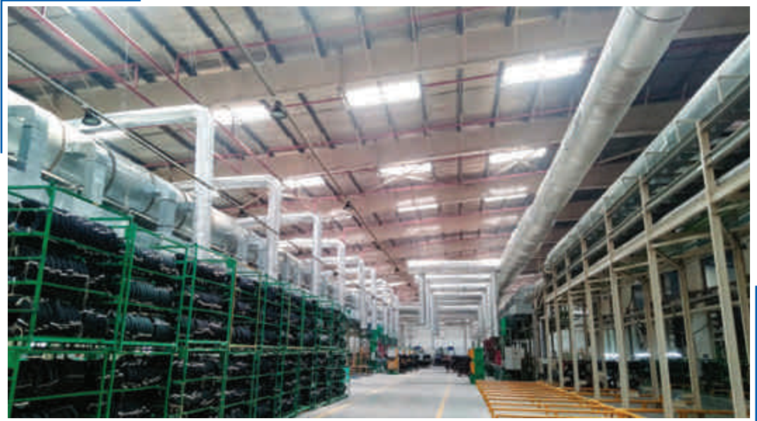
HVAC project at CEAT's tyre manufacturing facility at Nagpur
