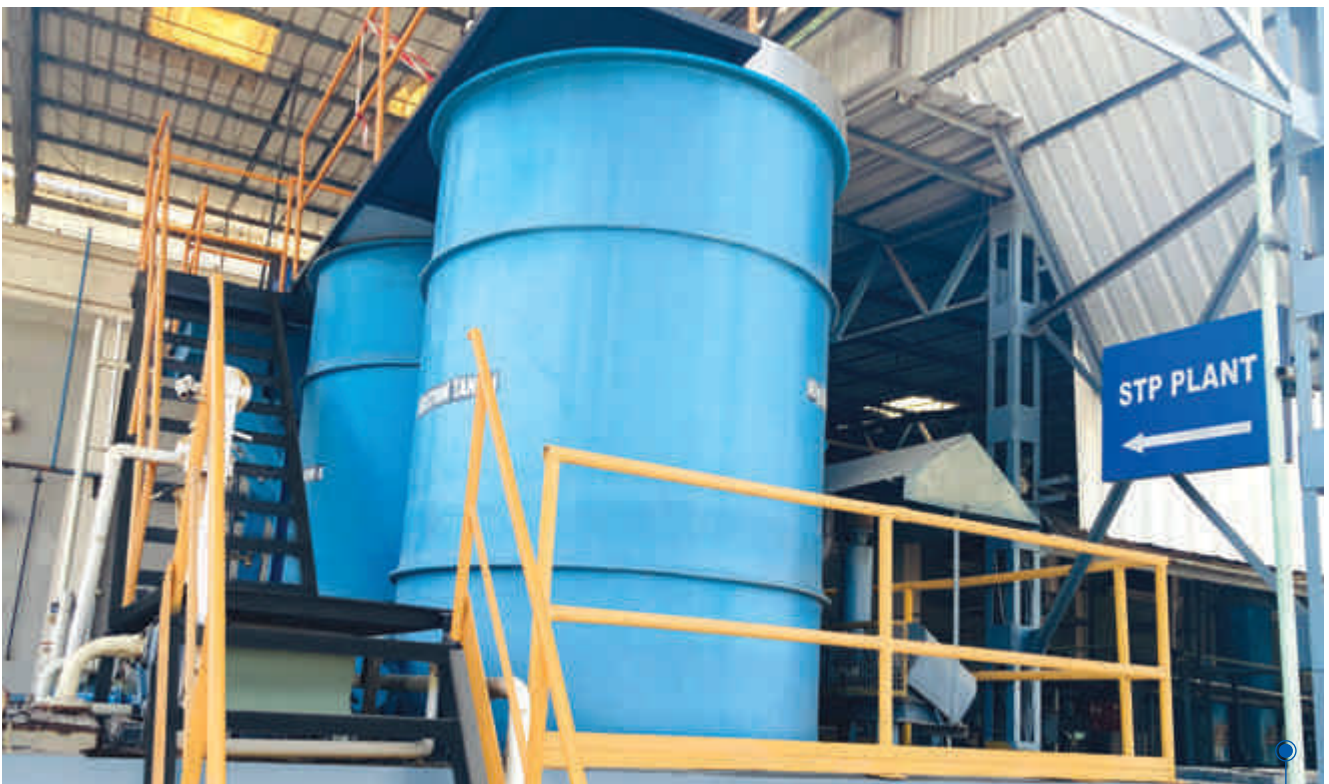
Sewage Treatment Plant (STP) at Blue Star's Dadra manufacturing facility
