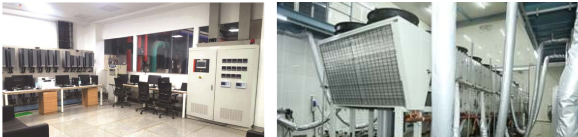
A glimpse of the control room (left) and test chamber (right) of the test facility where an air cooled chiller is being tested
