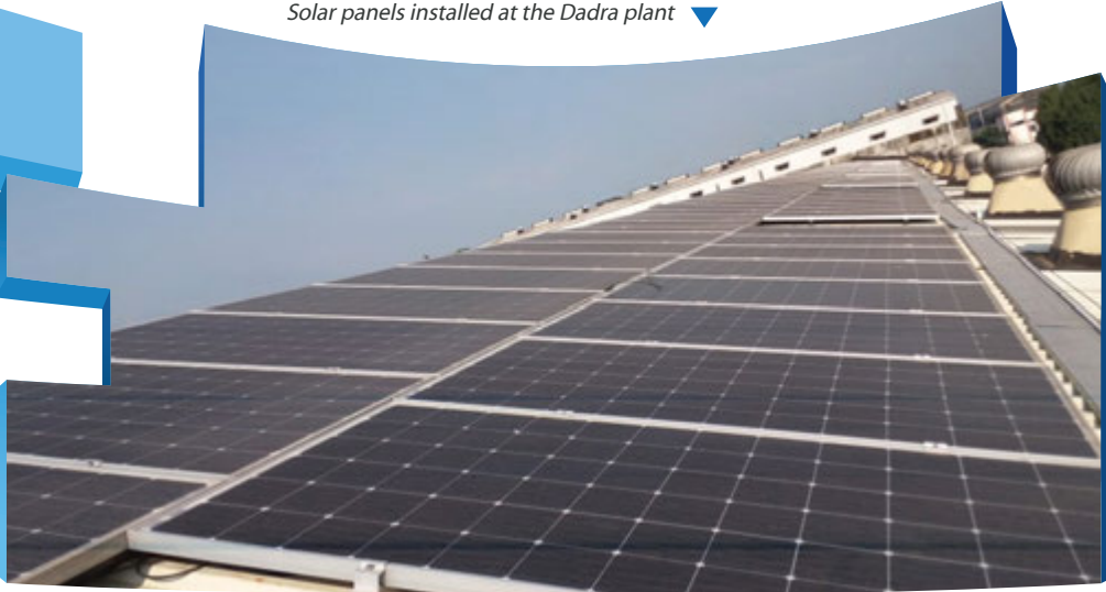
Solar panels installed at the Dadra plant ▼
