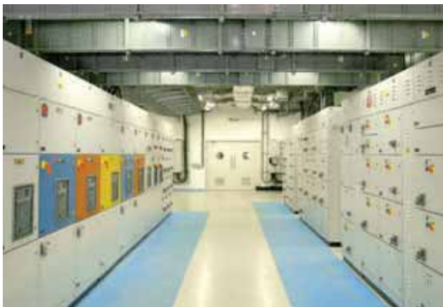
Mechanical, Electrical and Plumbing Systems for Dr Oetker, Rajasthan
