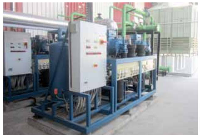
Refrigeration System for Hatson Agro Products, Chennai
