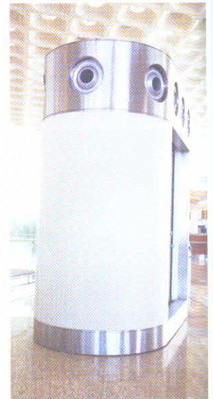
Photo 8: An air tower with jet nozzle outlets in the security hold area
