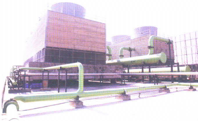
Photo 7: Cooling tower cells 2500TRx6
