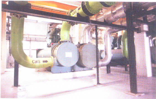
Photo 1: 2500TR centrifugal chillers with interconnecting piping
