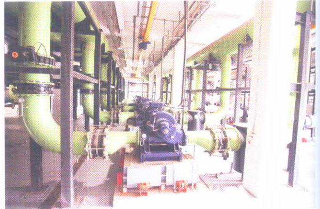
Photo 6: Condenser water pumps with 1300mm headers
