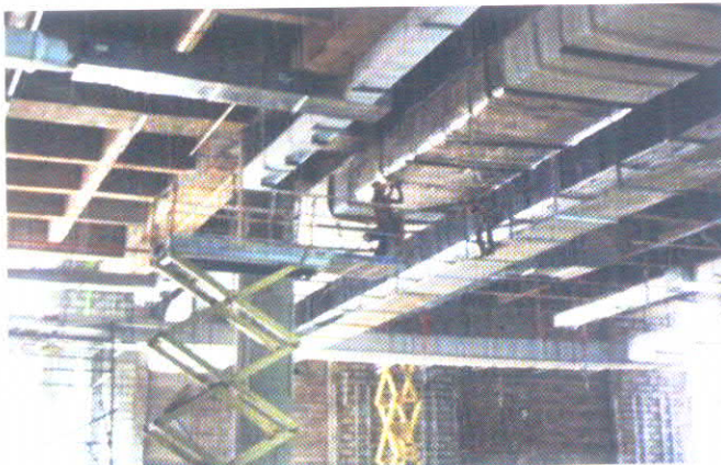
Photo 9: Ducting and insulation work in progress in immigration area with battery operated scissor lifts
