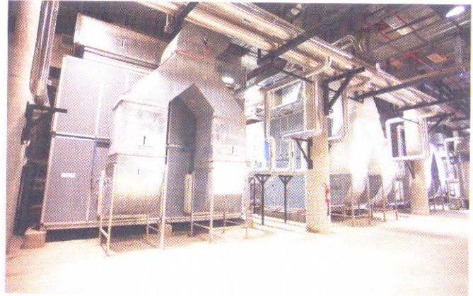
Photo 2: AHU duct and pipe connections
