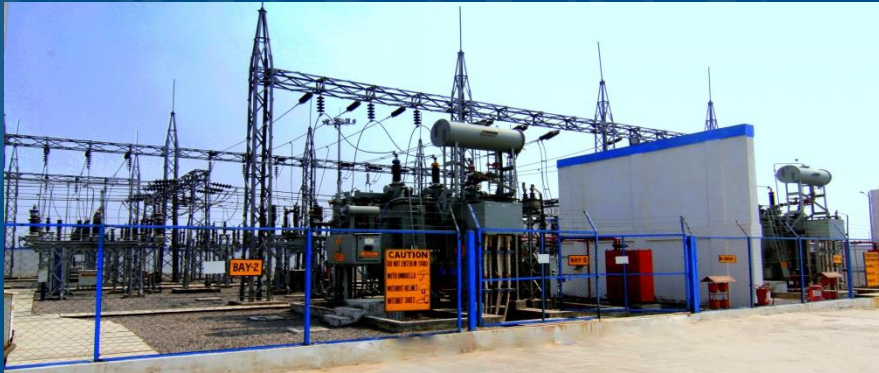
Tata Power - HT Substation
