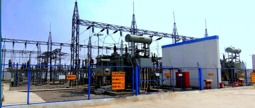
Tata Power - HT Substation
