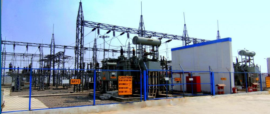
Tata Power - HT Substation
