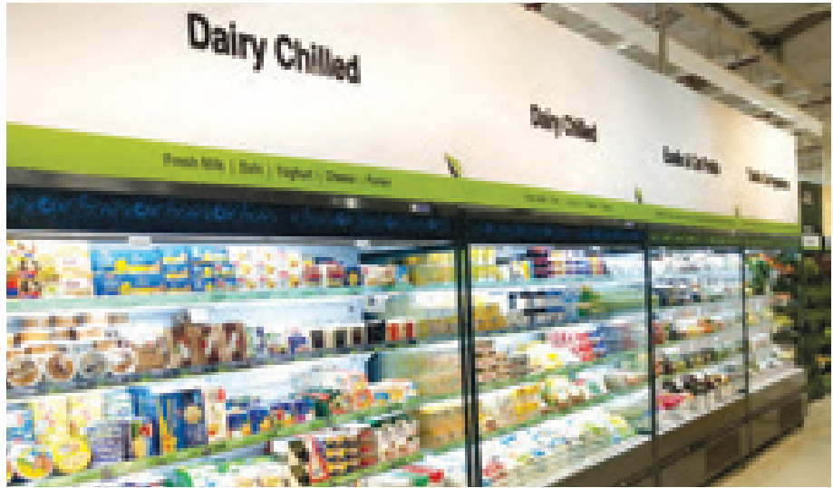
Supermarket refrigerators installed at Reliance Retail outlets across India
