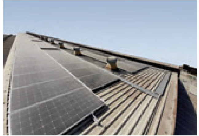
Solar Panels installed at Dadra Plant
